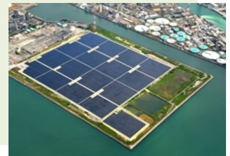
Megasolar power plant (to start operating in July 2014)
