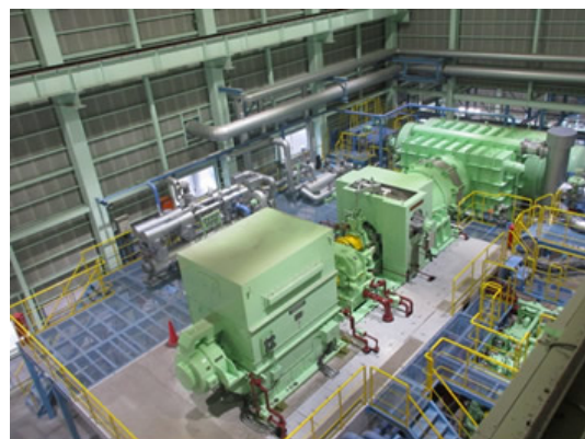
Exhaust heat recovery system at Kanda Factory
