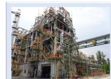
Second PCD manufacturing facilities in Thailand
