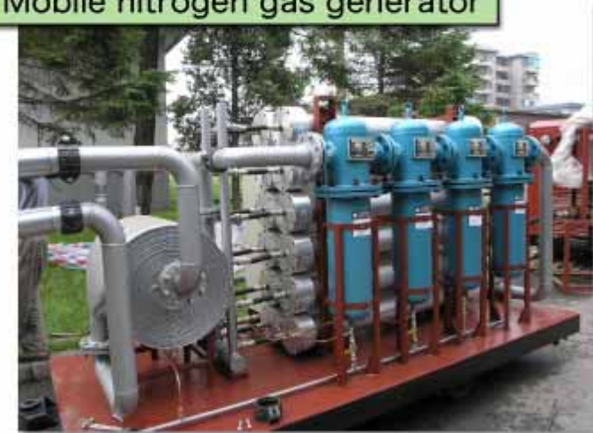
Mobile nitrogen gas generator
