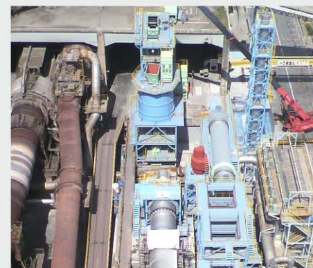
Waste plastic fuel conversion facilities (Kanda, Fukuoka)
