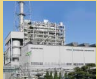
IPP power plant
